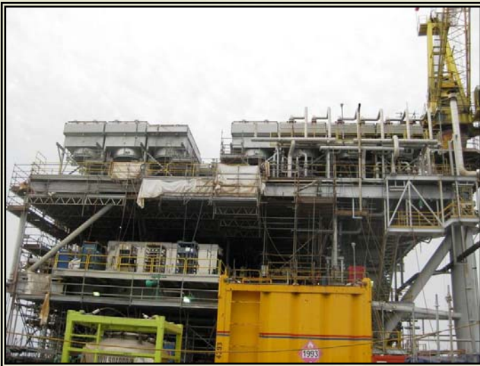
Above: New Turbine and Coolers
